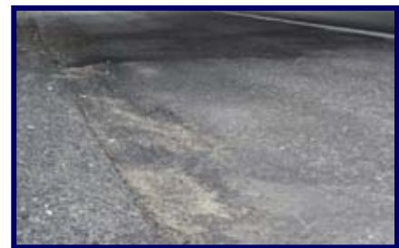
Figure 3 Drainage and Pavement Concern at Overpasses
